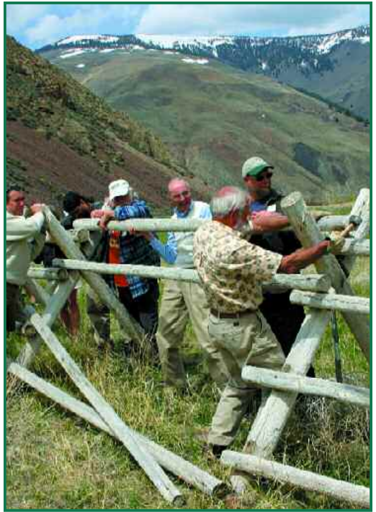
Retiring long-term WWP Board member Gene Bray leads the fence repair team at the May Board meeting at WWP's Greenfire Preserve
